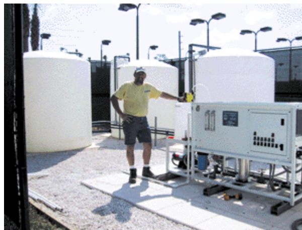
Dave Silverman stands near a commercial RO system his company installed.
